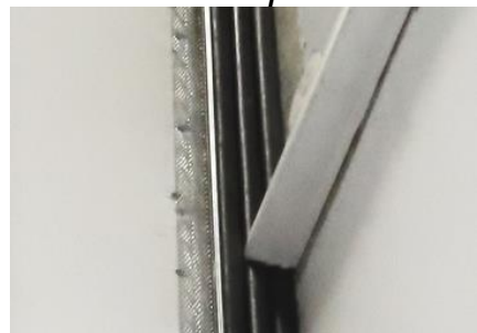
Precast Panel insulation was cut on eitherside of the partition and the silicone/foam joint is installed properly
