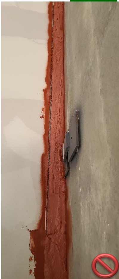
The fire rated joint exceeded the capability of the fire spray and seperated at the drywall partition.
